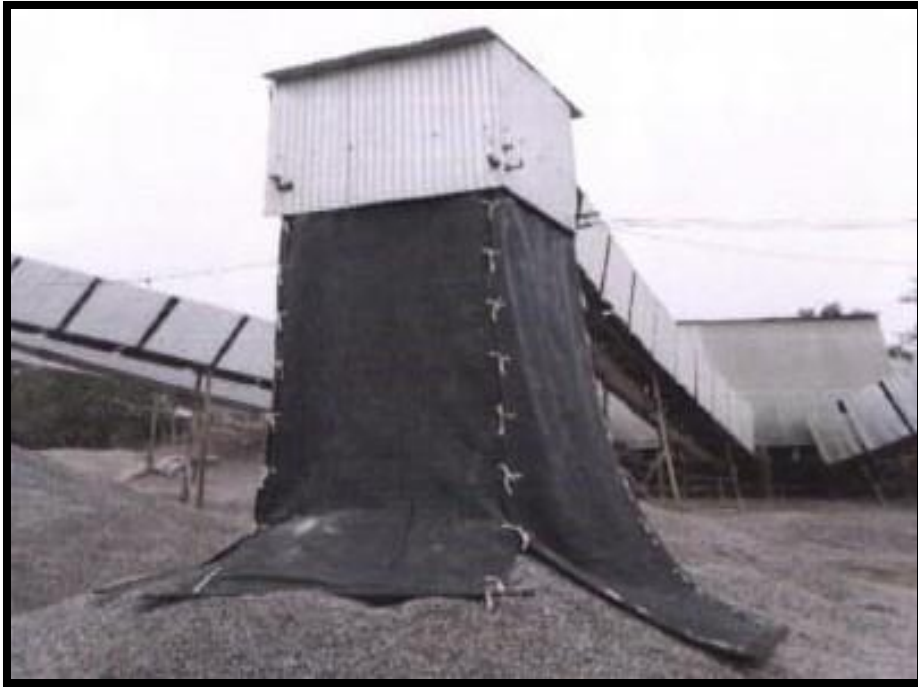
Figure-2: Chute from top of discharge point
